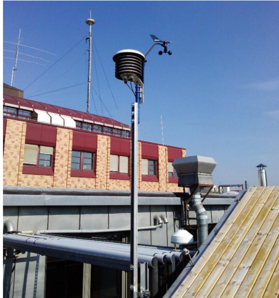
Fig. 4. Weather station on the roof top.
