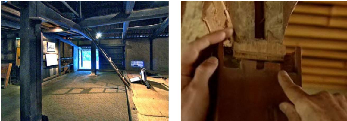
Figure 03: Highly flexible kit system Left: Interlocking Technology: beams and columns of a traditional Japanese house were only plugged together and the joints allowed the joined elements to move within a certain scope. (1) Right: Backbone Technology: a middle column frame or a central pillar forming a kind of backbone of the house which was fixed to the ground and the other columns were allowed to move on the foundation in case of vibrations. (1)
