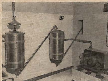
8) Milk storage room as part of a "Miele" stall-type milking system equipped with pre-cooler and low-temperature cooler (Miele & Cie.)
