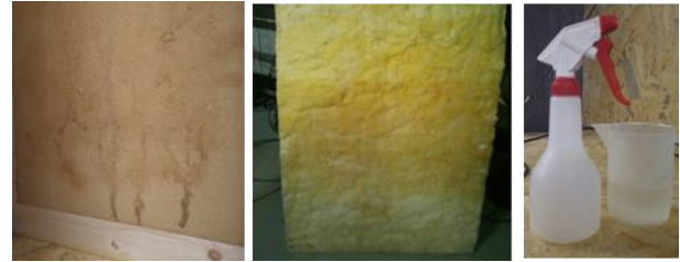
Figure 7: Wet wood fiber board (left), wet mineral wool (middle), spraying equipment (right)
