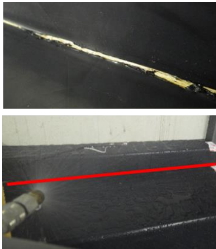
Figure 11: Cut in the second defence layer and spray water on the cut
