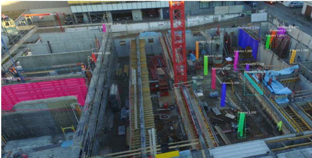
Figure 14: Formwork and column elements detected by a trained CNN using Mask R-CNN on Test Site C
