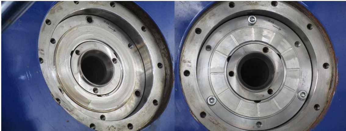
Figure 4: left: damaged turbo generator rear bearing showing completely removed lubricating channels, right: new installed bearing with lubricating channels
