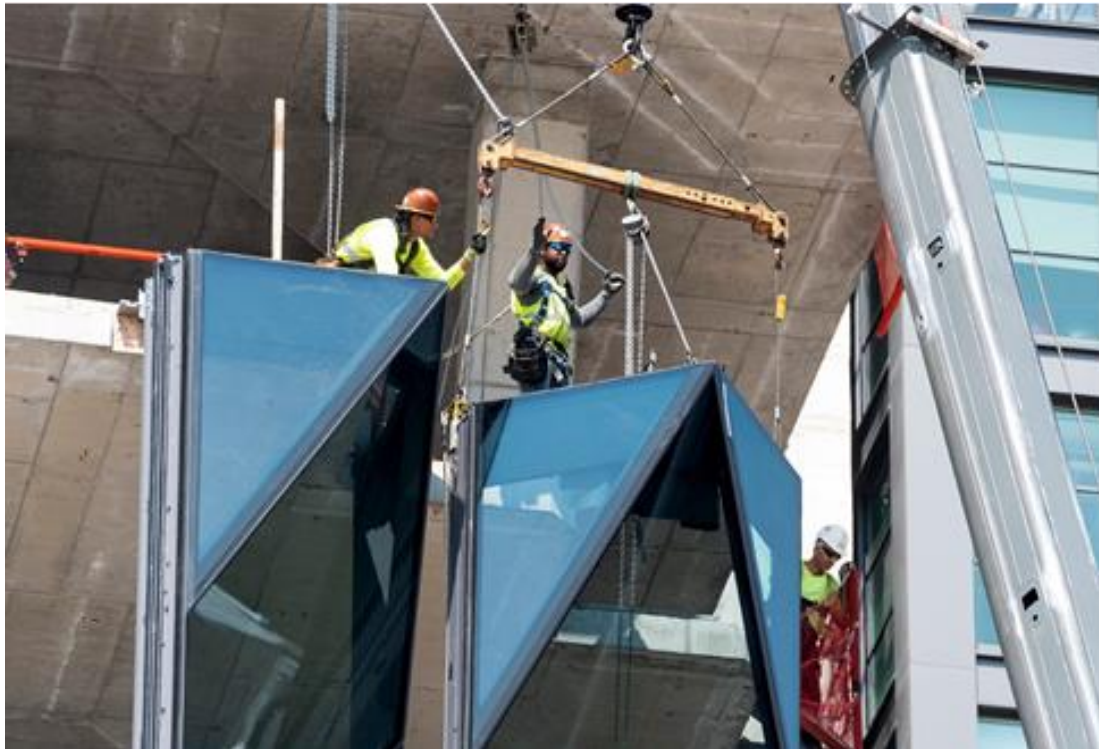
Figure 4-4: Several workers working at height during the CWM installation process (facade installation in Solar Carve Tower, New York. Facade engineered and manufactured by Focchi Group; photo by Timothy Schenck).
