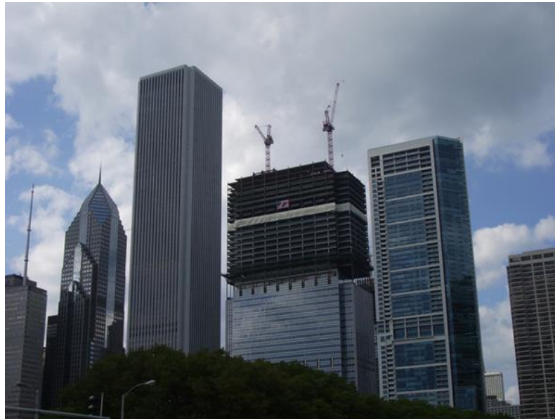
Figure 6-6: Blue Cross Blue Shield Tower in Chicago during expansion. Photo by Photogal (unchanged and licensed under CC BY-SA 3.0, https://creativecommons.org/licenses/by-sa/3.0/ )
