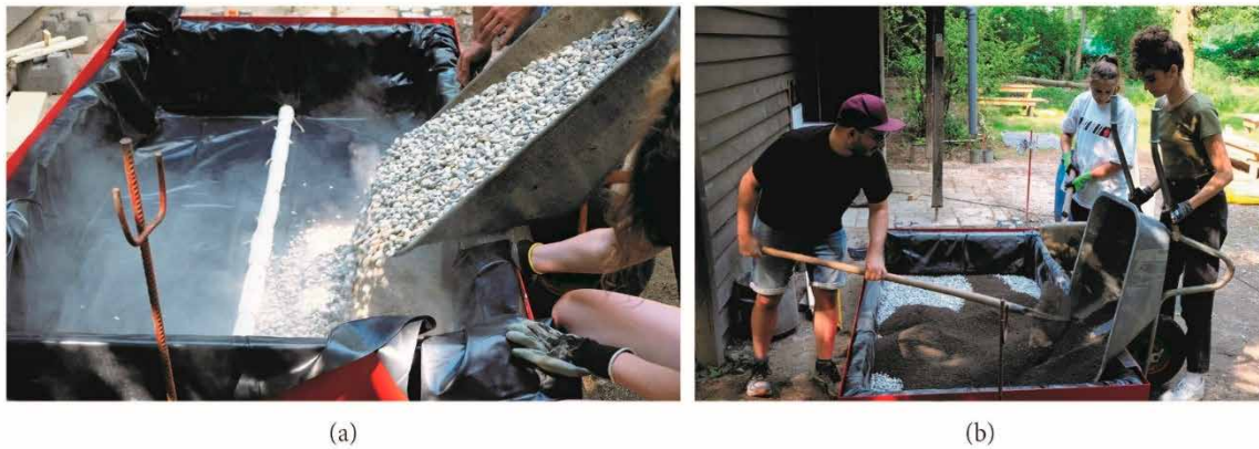
Figure 13. Construction work on the filter trough. (a) The drainage layer consists of 15 cm of gravel. (b) A layer of lava sand follows the gravel.
