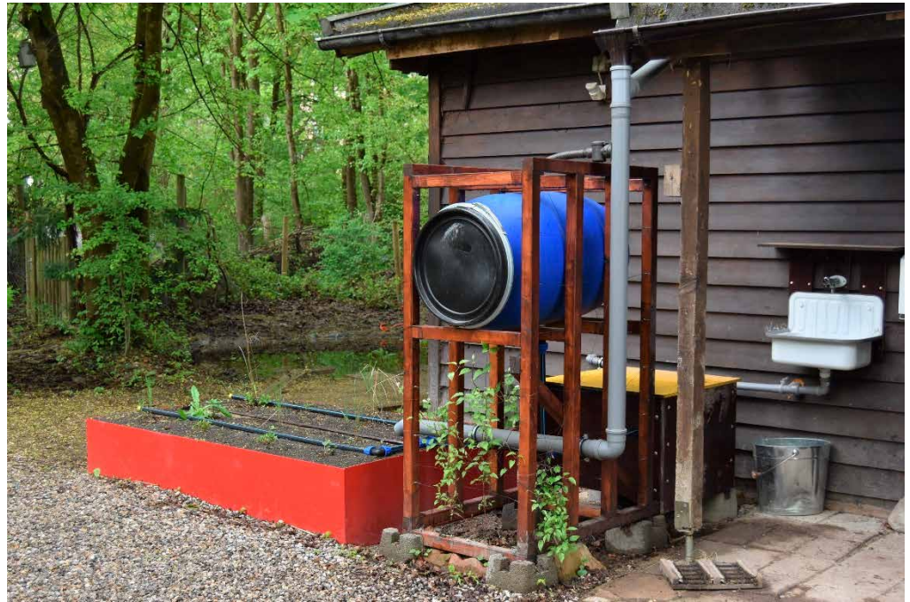
Figure 14. Built result of the BGA project 10 months after completion. The operation ran without any disruptions. In winter, the septic tank was bypassed. In the meantime, summer operation was resumed. The plants on the constructed wetland all survived the winter well and will grow even bigger in the next few years.
