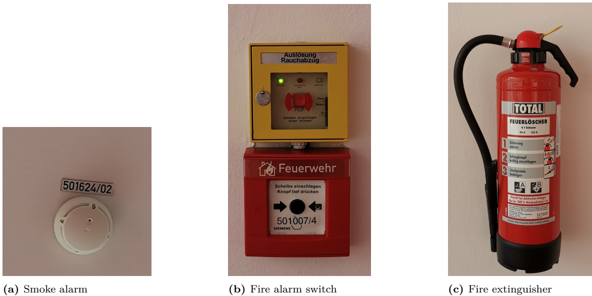
Figure 1.4: Fire safety equipment
