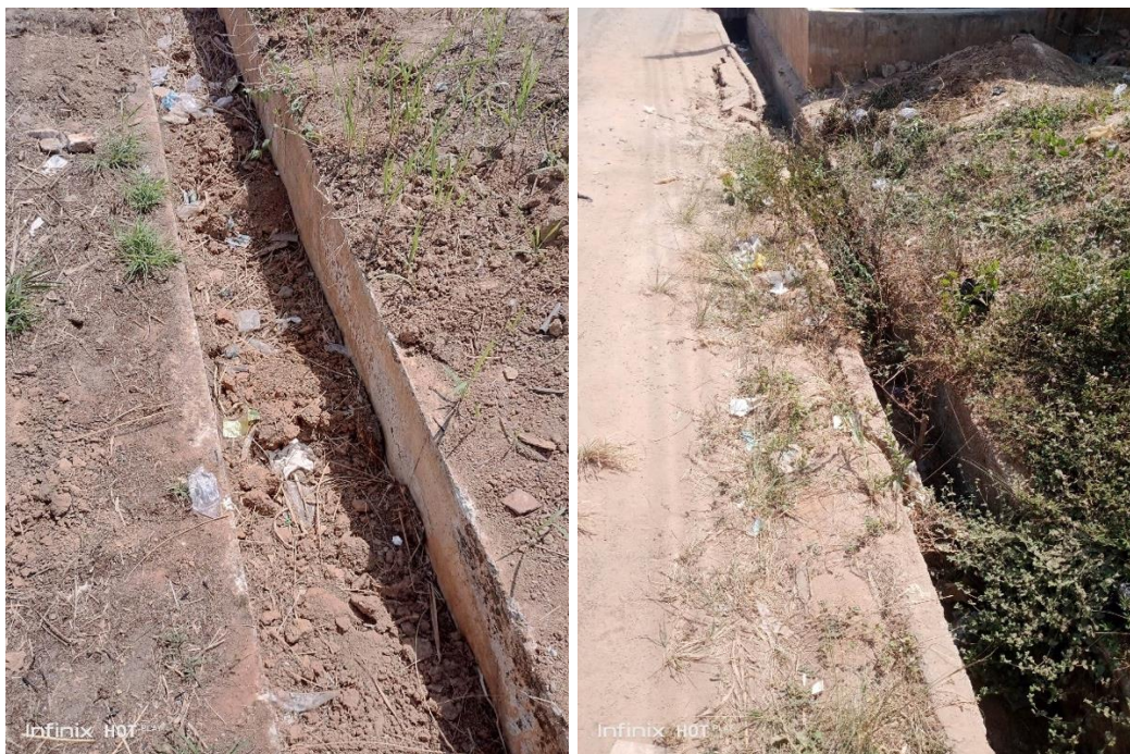
Figure 62: images of blocked drainage channels (Author, 2023)
