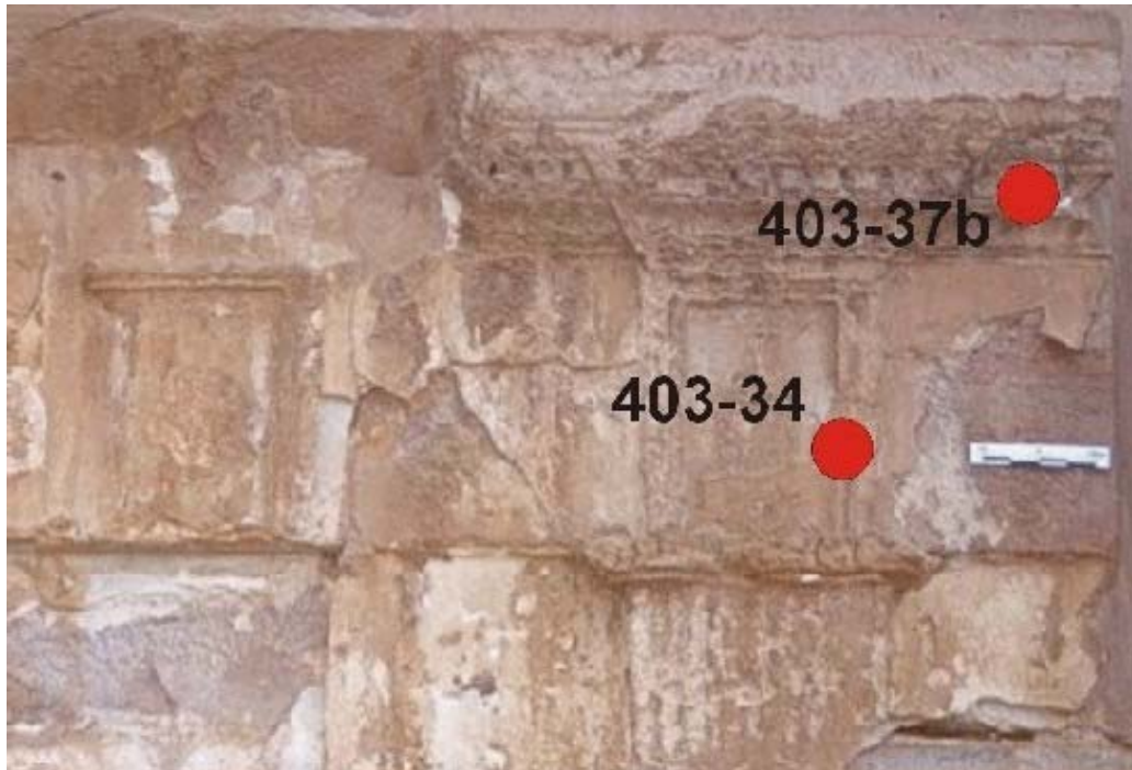
Figure 83. Sampling of the stucco on the right side of the southern façade.
