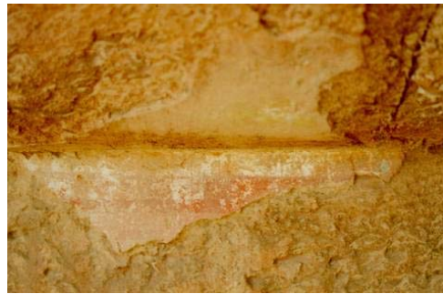
Figure 20. Red and white paint on fascia.
