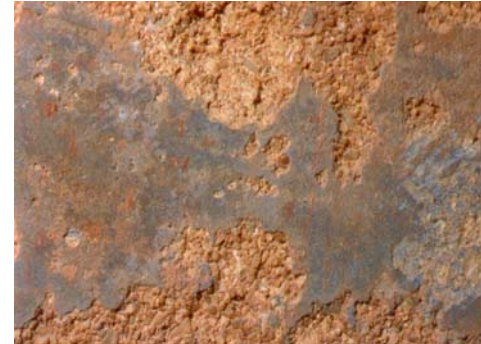
Figure 24. Detail of blue paint on fascia.
