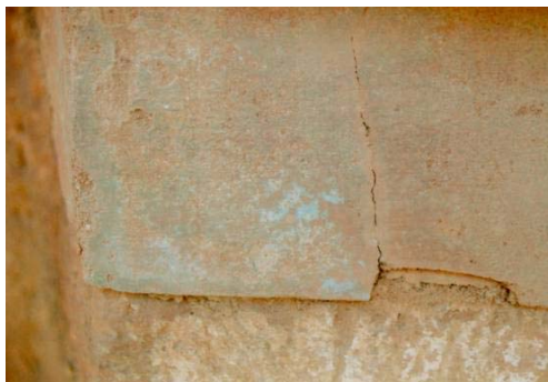
Figure 23. Blue paint on fascia below torus.
