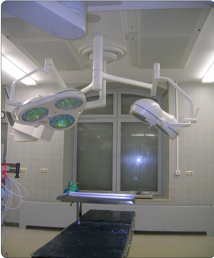
Figure 8.3: OP I: Two rectangular ventilation inlets are placed at the ceiling around the area of the operating table. The velocity of the instreaming air is adjusted to 0.24 m/s which corresponds to a ventilated air volume of 2780 m 3 /h.
